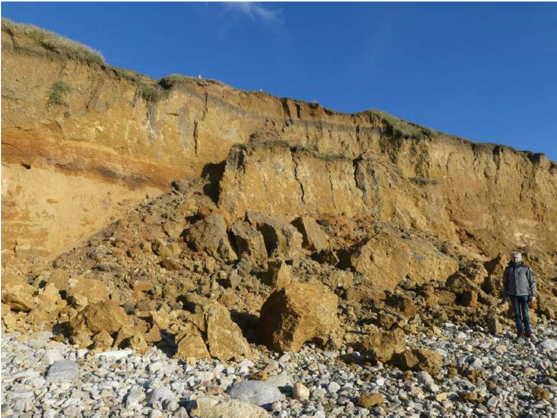
Eboulement à Pen Had © S. Coat RNR 14/01/2026
